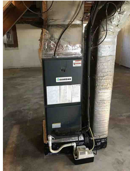
HVAC air handler
