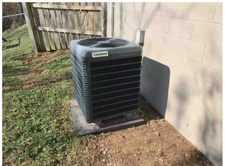
HVAC condensing unit
